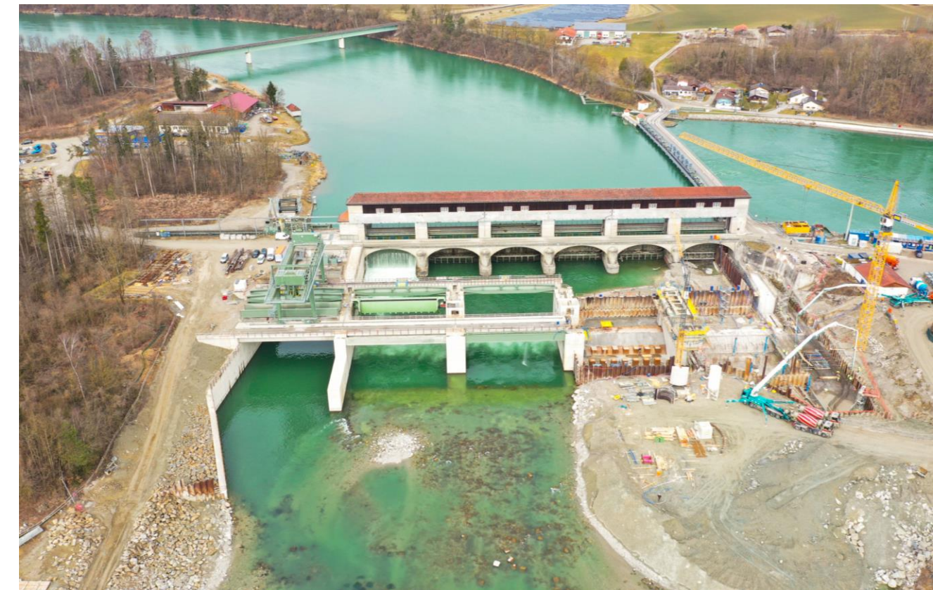
Power plant Töging (DE)
